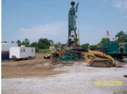
Injection well drilling at test site for geologic sequestration of carbon dioxide in the study area
