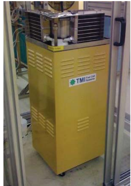
1 kilowatt SOFC genset operating at Lockheed Martin, running on DoD standard JP-8 fuel
