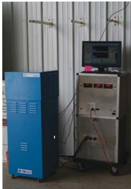
1 kilowatt TMI solid oxide fuel cell running on soybean oil during a 30-day, on-farm demonstration in Wakeman, OH
