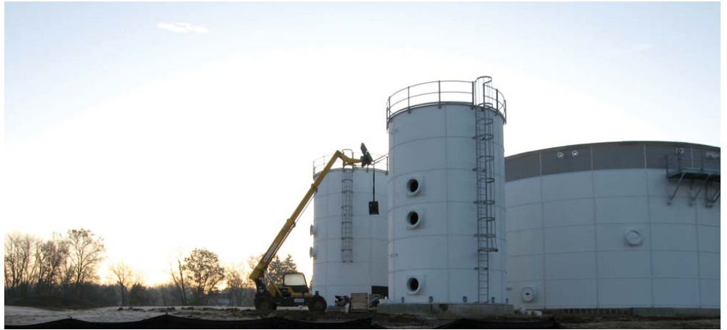
Waste-to-energy project under construction at The Ohio State University Ohio Agricultural Research and Development Center in Wooster.
